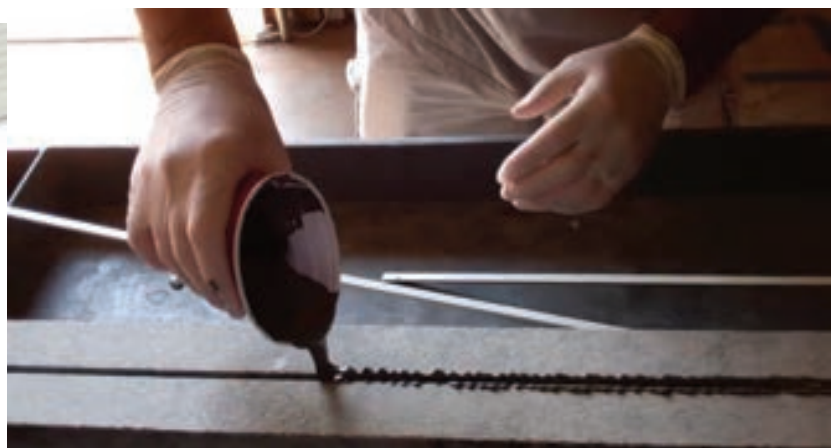
Epoxy being poured into the back of the slab before inserting rods
